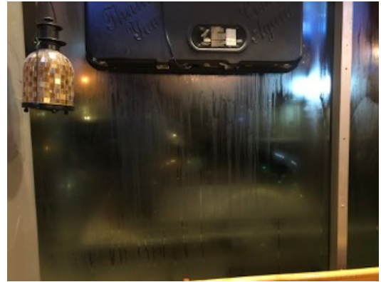
Condensation on window interiors
