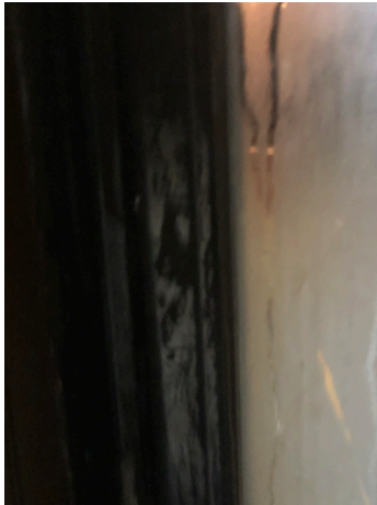
Interior ice buildup due to frozen condensation
