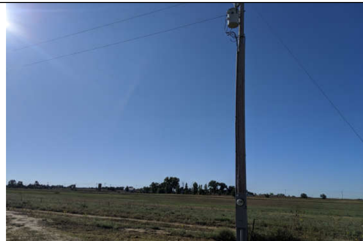
Description: Distribution lines on south side of Site. Direction: Southeast
