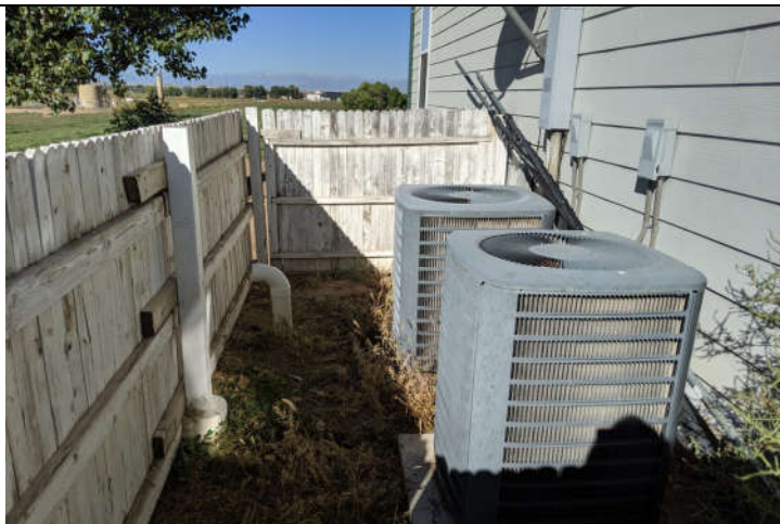
Description: Cooling system on south side of west residence. Direction: West
