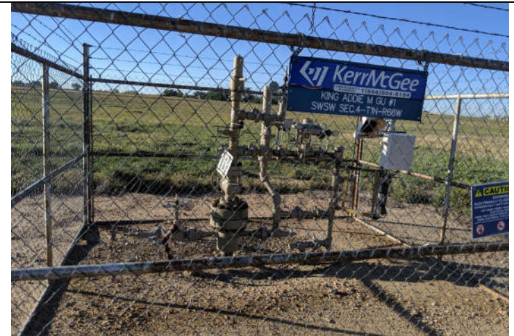
Description: Kerr McGee oil and gas well; de minimis staining. Direction: South
