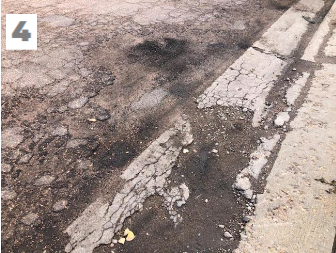
4. The damaged street gutter in front of Mahnke's work bay on Sixth Street.
